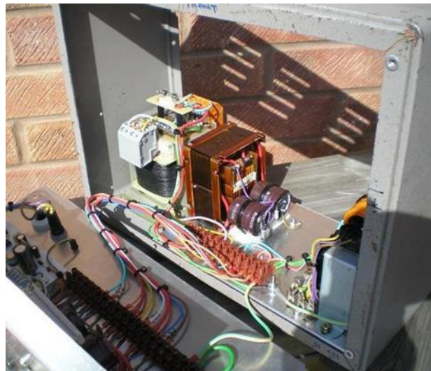
Figure 6. Power supply components in the base of the case. A shadow of the ventilation slots in the top is seen on the wall behind the case
